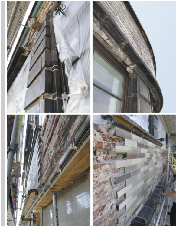
Figure 10. Conservation works at the facade of Renoma department store. Top left: fourth floor pillar finished with a flower finial. Top right: attic wall at the corner of the building with corroded sleepers and cornices. Bottom: renovated fragments of the northern facade. As in 2008. Photo by P. Kirschke
